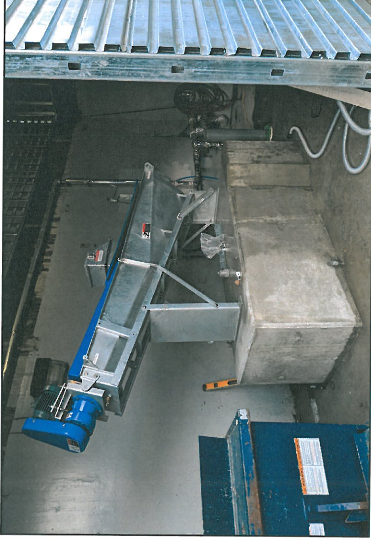
Grit classifier at Snoqualmie, WA WWTP
