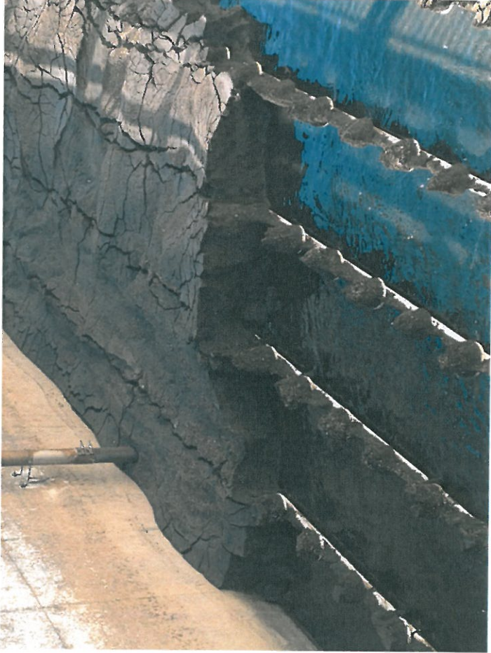
EXAMPLE OF GRIT BUILD UP IN AN AERATION BASIN
